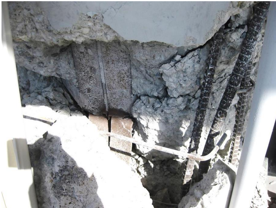
Figure 10: Fracture at weld
