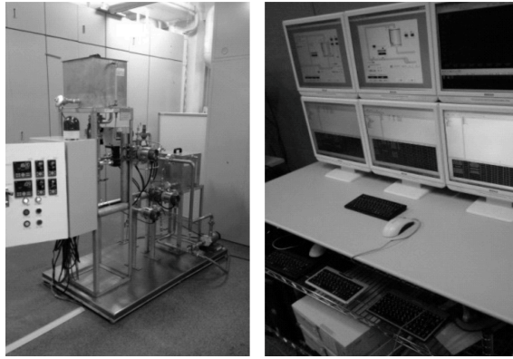
Figure 5.2: The plant side (left) and the operator side (right) of the testbed. Testbed visitors can operate the system during the demonstration.
